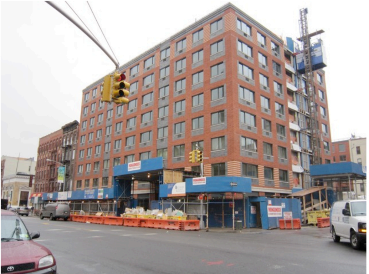
The Douglass, a building for low-income renters is under construction at the corner of Frederick Douglass Boulevard and West 128th Street in Harlem. (DNAinfo/Jon Schuppe)
